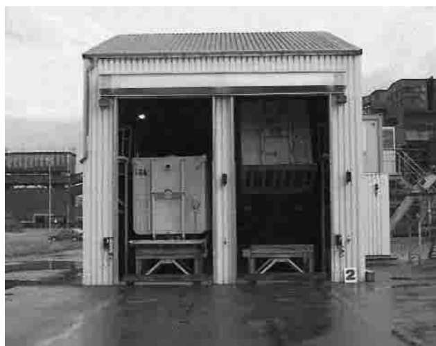
Fig. 6 – Plastics unloading station at blast furnace 1, container tipping station.
